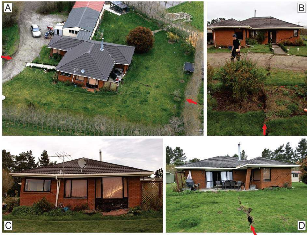
Figure A2.10 Telegraph Road house and Greendale Fault surface rupture; see Figures A2.7 and A2.8 for location. Red arrows denote location of discrete surface fault rupture. (A) Aerial view looking south. Photo by Richard Cosgrove. (B) View looking west-northwest. Photo by Hayden Mackenzie. (C) View looking south-southwest. Photo by Hayden Mackenzie. (D) View looking east-southeast. Photo by Dougal Townsend.
