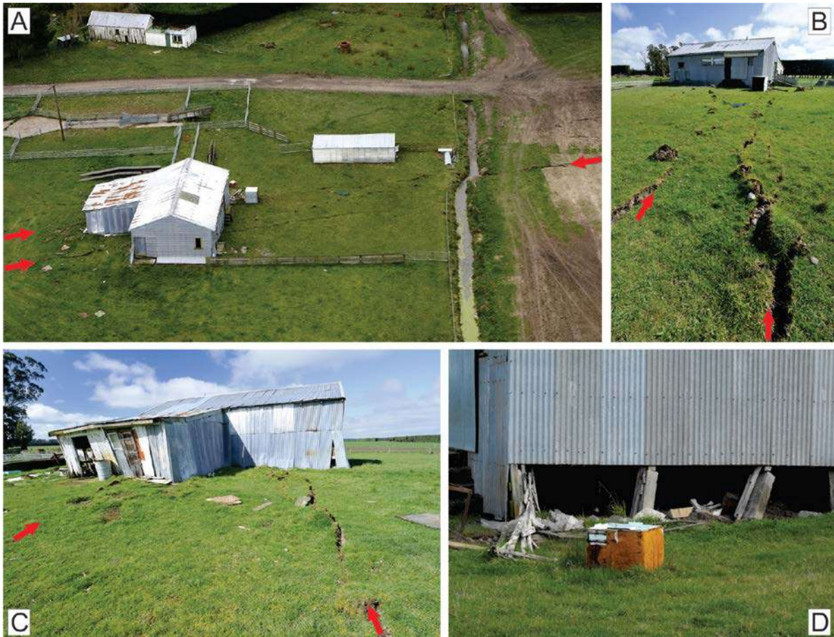
Figure A2.11 Kivers Road woolshed and Greendale Fault surface rupture; see Figures A2.7 and A2.8 for location. Red arrows denote location of discrete surface fault rupture. (A) Aerial view looking northeast – note dextral offset of irrigation channel in right-hand side of photograph. Photo by Richard Cosgrove. (B) View looking west. Photo by Dougal Townsend. (C) View looking east. Photo by Dougal Townsend. (D) View looking southwest showing detail of shallow-seated concrete piles. Photo by Russ Van Dissen.
