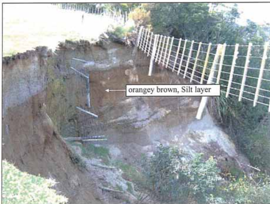
Fig. 2: Slip scarp along the south-western side of the subdivision displaying the distinct stratification of the volcanic soils.
