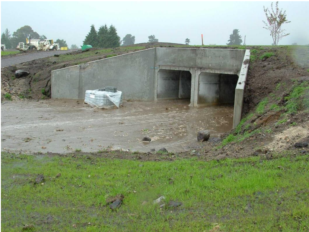
Loch Eagles Subdivision, 2013. Large volume of pumice debris following a downpour during subdivision development.
