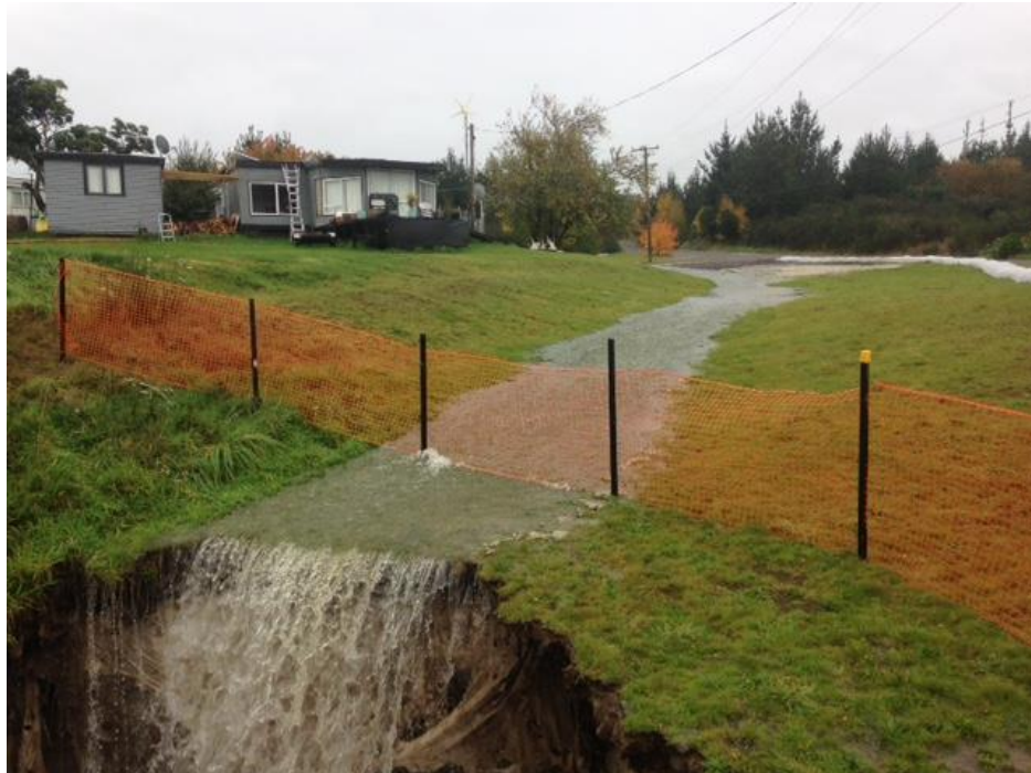
Paenoa Road, Acacia Bay, May 2017. Cyclone Debbie. Overland flows and gully erosion of geotechnically protected area.
